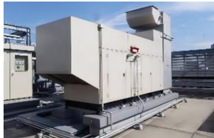
Emergency power facility
