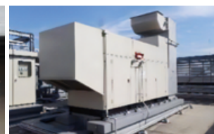
Emergency Power Facility
